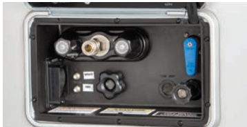
Water and utility management center
