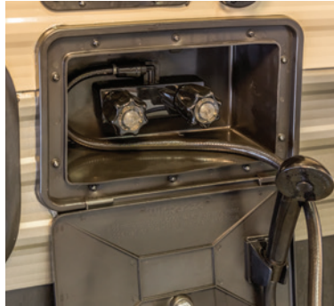
Outside Shower with Hot and Cold Water
