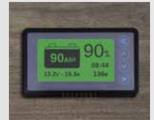
Upgraded battery monitor displays battery statistics like amp-hours consumed, state of charge, and voltage.
