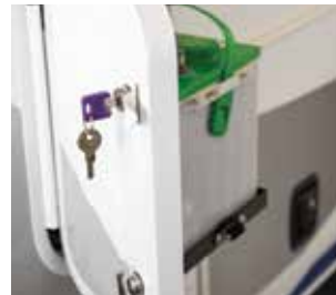
Lockable weather resistant battery compartments also prevent theft. N/A 1475 & 1575
