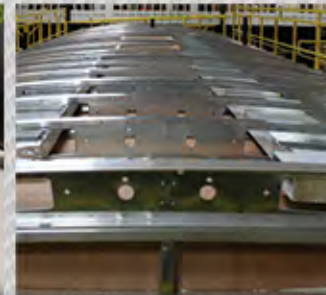
Walkable steel truss roof system
