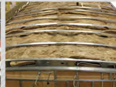
Aluminum truss roof system
