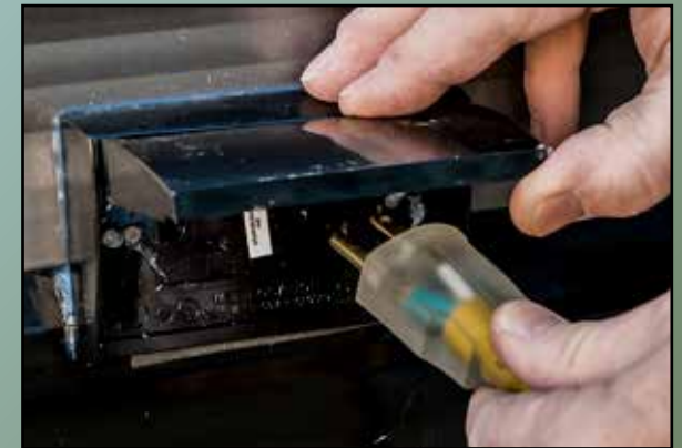
Convenient Outside GFCI Protected and Covered Outlet.
