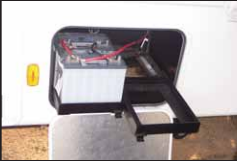
Slide out battery trays come with 2 batteries and room for two more.
