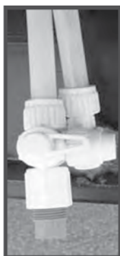
Water Tank Drain Valve
