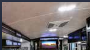
Dual Ducted A/C System
