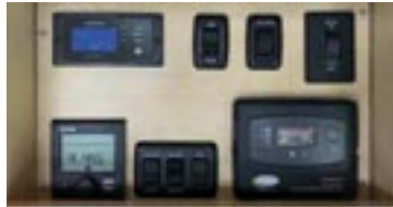
Convenient control center monitors capacities
