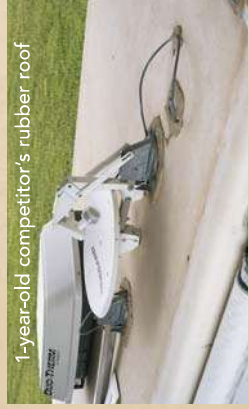
1-year-old Itasca fiberglass roof
