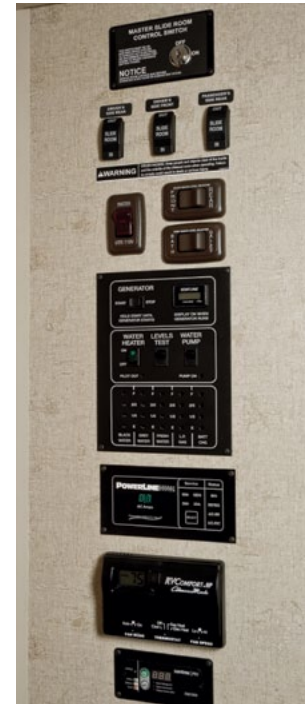
Power Protector The OnePlace® Systems Center houses the PowerLine® Energy Management System (35B, 35F), which minimizes tripped campground circuits during periods of heavy usage.
