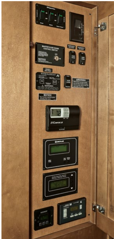
Important gauges, switches and controls are all centrally located in the OnePlace® Systems Center .
