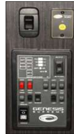
Centralized Monitor, Lighting & Inverter Controls
