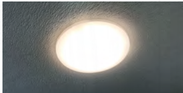
LED Interior Lights
