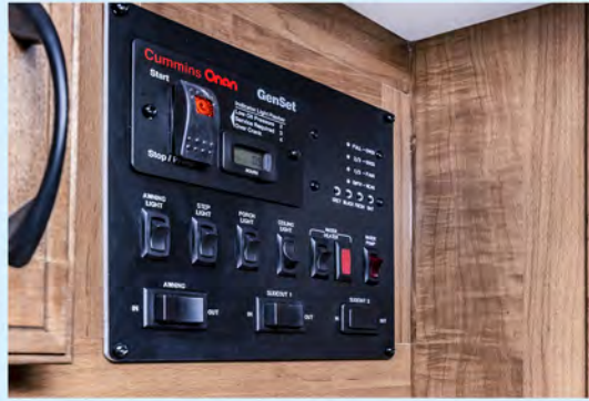
▲ Located just inside the entry door, the control panel includes switches for generator, slide-outs, lights, awning, and other power features.
