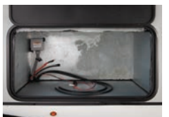
Generator Prep (Standard 27KB, 29SS)
