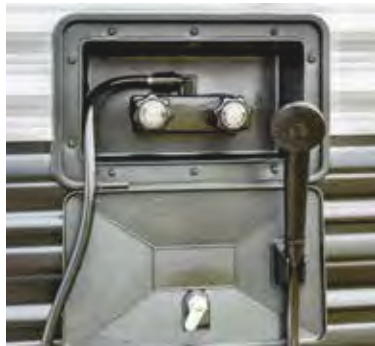
Outside Shower with Hot and Cold Water
