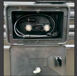
Outside Shower with Hot and Cold Water
