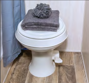
Foot Flush Toilet
