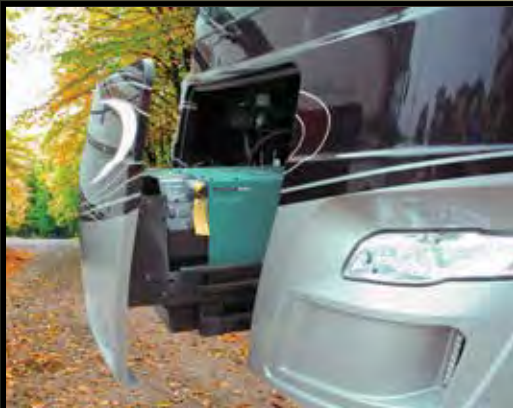
SLIDE-OUT GENERATOR TRAY
