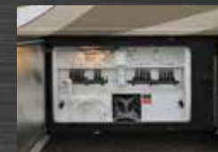
Berkshire's water manifold system with whole unit filter and exterior shower.
