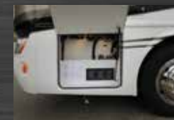
Easily accessible electrical fuses with Berkshire's no fuss schematic.
