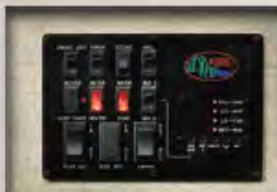
SIERRA's control center allows you to monitor tanks and other systems quickly and easily.
