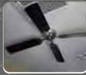
Two (2) Ceiling Fans (Bedroom and Living Area)
