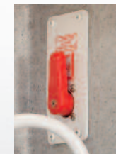
Hot water bypass valve
