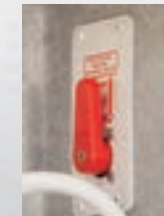
Hot water bypass valve
