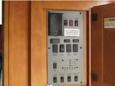
Central control panel with light and slide switches, tank monitors, awning, water heater and pump controls.
