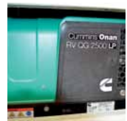
Propane Generator for charging your batteries, running the A/C or other 110 volt devices
