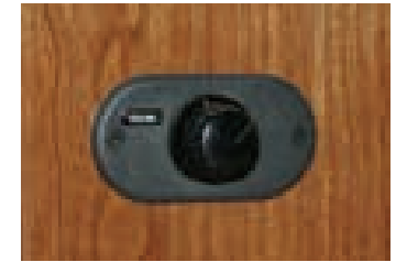
Dimmer switches selectively control LED lighting zones.
