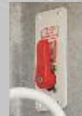
Hot water bypass valve
