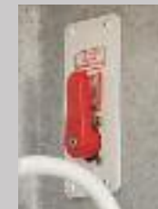
Hot water bypass valve
