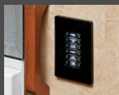
Multi-Plex lighting system touch control.
