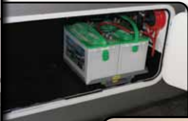
Four compartment battery storage.
