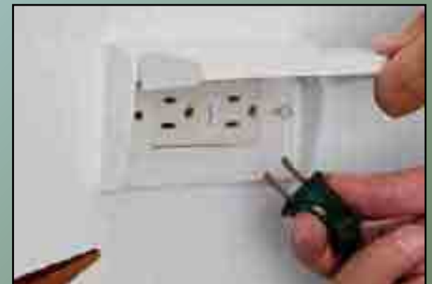
Convenient Outside GFCI Protected and Covered Outlet.
