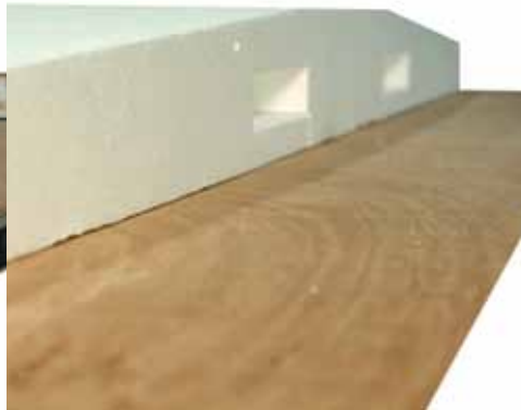
Radius roof foam with built in A/C ducts
