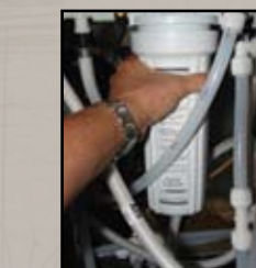
The city water fill is filtered. Cartridges can be changed through an access hatch
