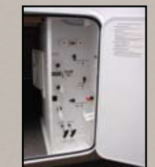
The convenience center provides access to all major plumbing functions and the enclosed dump valves
