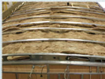
Aluminum truss roof system
