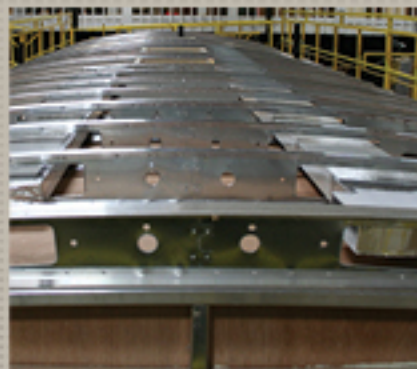
Walkable steel truss roof system
