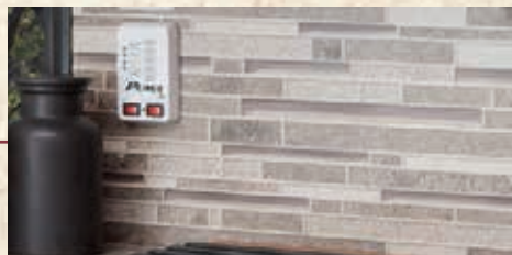
Decorative backsplash with monitor panel that indicates battery strength, tank capacity and water pump details.
