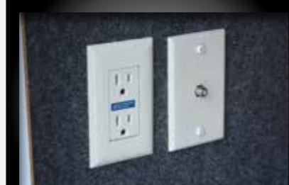
110v outlet and cable outlet conveniently located in the pass-thru storage area.
