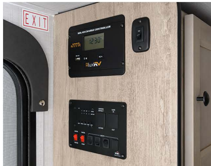
Below: Systems Control Panel & Solar Charge Controller (160FK shown)
