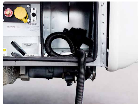
Macerator Sewage Discharge With Manual Disconnect
