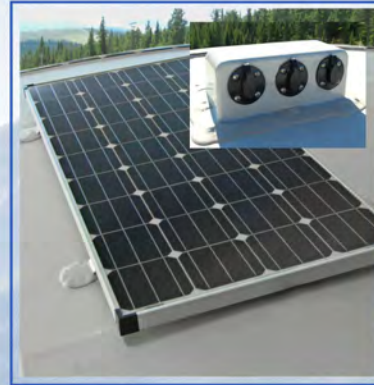
170 Watt Roof Mounted Solar Panel
