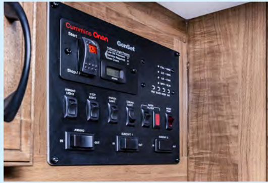
▲ Located just inside the entry door, the control panel includes switches for generator, slide-outs, lights, awning, and other power features.
