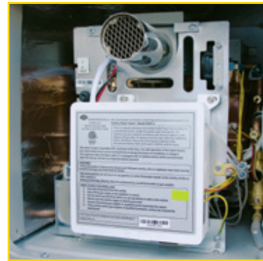
Tankless Water Heater
