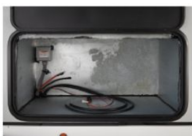
Generator Prep (Standard 27KB, 29SS)
