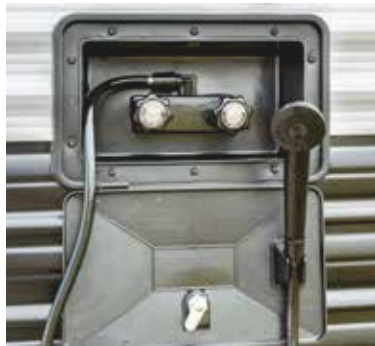
Outside Shower with Hot and Cold Water
