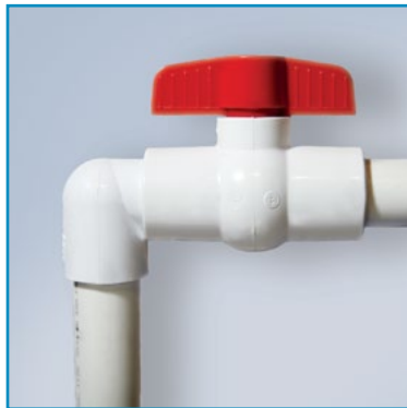
1" Fresh Water Tank Drain
