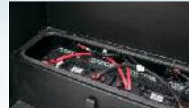
Two batteries in a single housing for easy access. (One battery LE and Transit)
