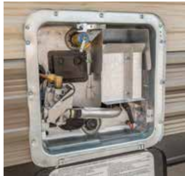
5 Gallon Water Heater
