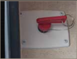
Battery disconnect in pass thru storage
