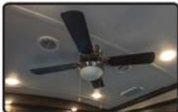
RESIDENTIAL CEILING FAN PROVIDING NATURAL AIR MOVEMENT
