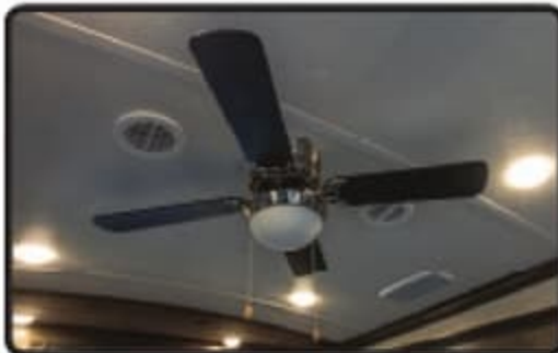
RESIDENTIAL CEILING FAN PROVIDING NATURAL AIR MOVEMENT
